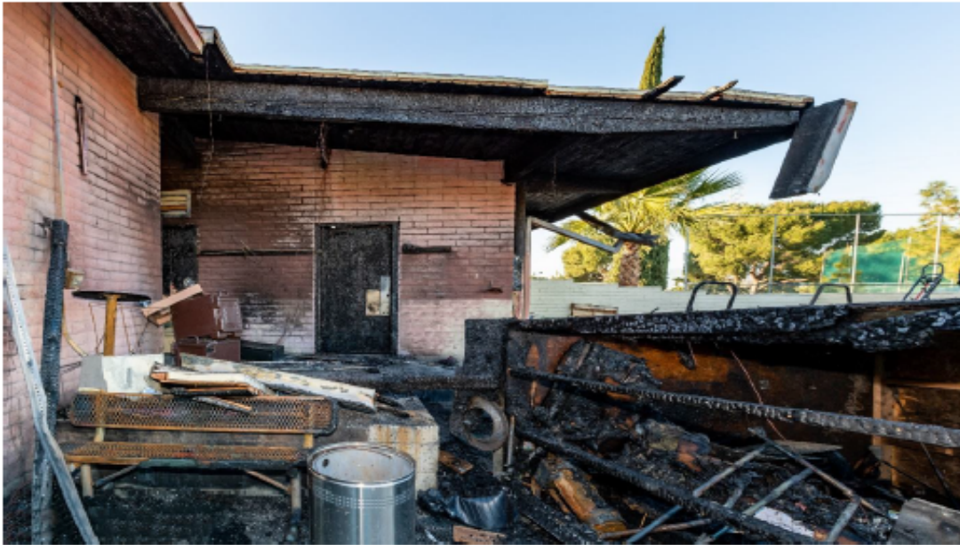
Photos of Fire Damage
